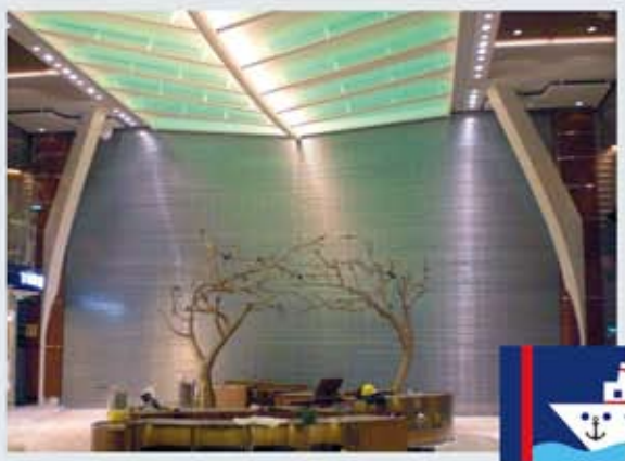
Fire protection roller door A60 in a shopping center of a cruise liner 15 x 8,75m
